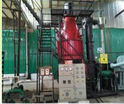
Producer Gas Unit
